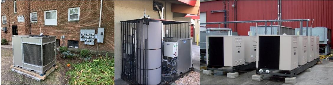
Figure 18: Commercial Installations of Sorption FFHP Equipment Including GTI Energy Demos in Multifamily Buildings (Left), Full-Service Restaurants (Center), and a Commercial Installation of Equipment (Source: GTI Energy/Robur)
