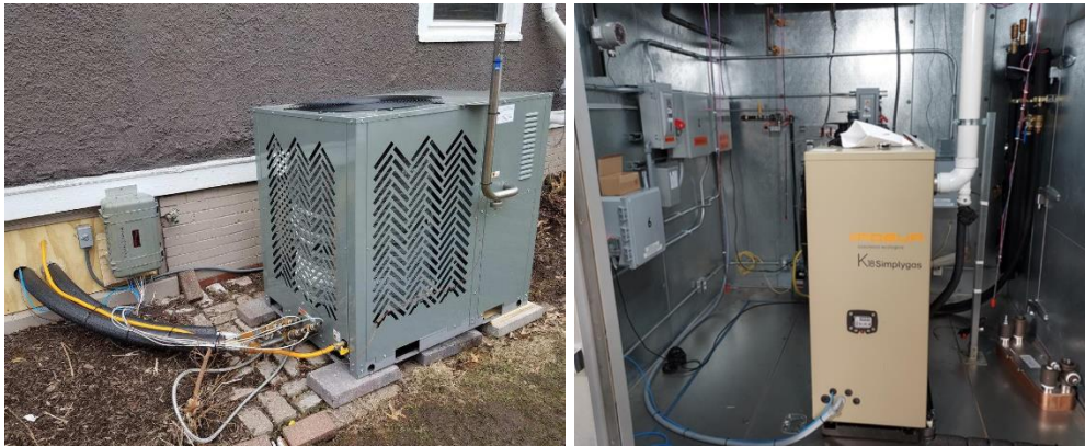
Figure 21: FFHP Installation Site for Hydronic Heat Distribution/Hot Water (Left) and Commercially-Available Residential FFHP at GTI Energy Laboratory (Right)
