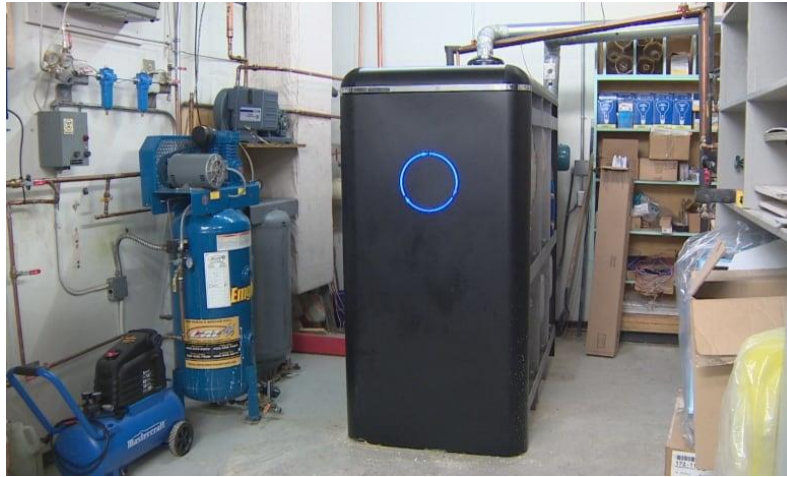
Figure 46: Installation of Manufacturer A's Carbon Capture Unit at Facility Owned by Canadian Utility [CBC, 2019]
