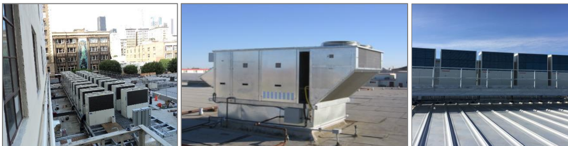
Figure 24: Installations of Multiple Vapor Compression-Type FFHPs (Source: Multiple Manufacturers)
