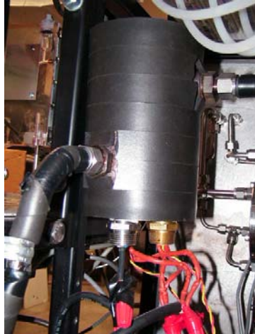
Figure 20 Heating section of spray water loop.
