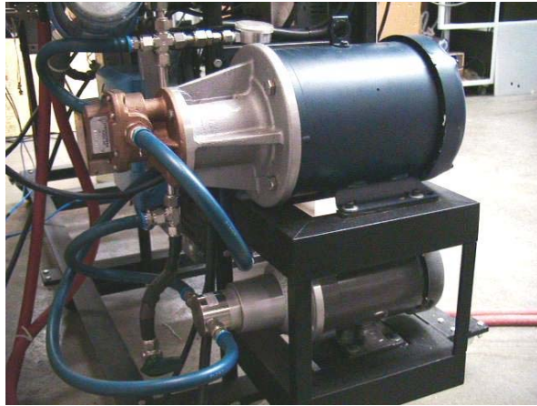
Figure 18 Stacked 1-hp and 3-hp pumps for spray water loop.
