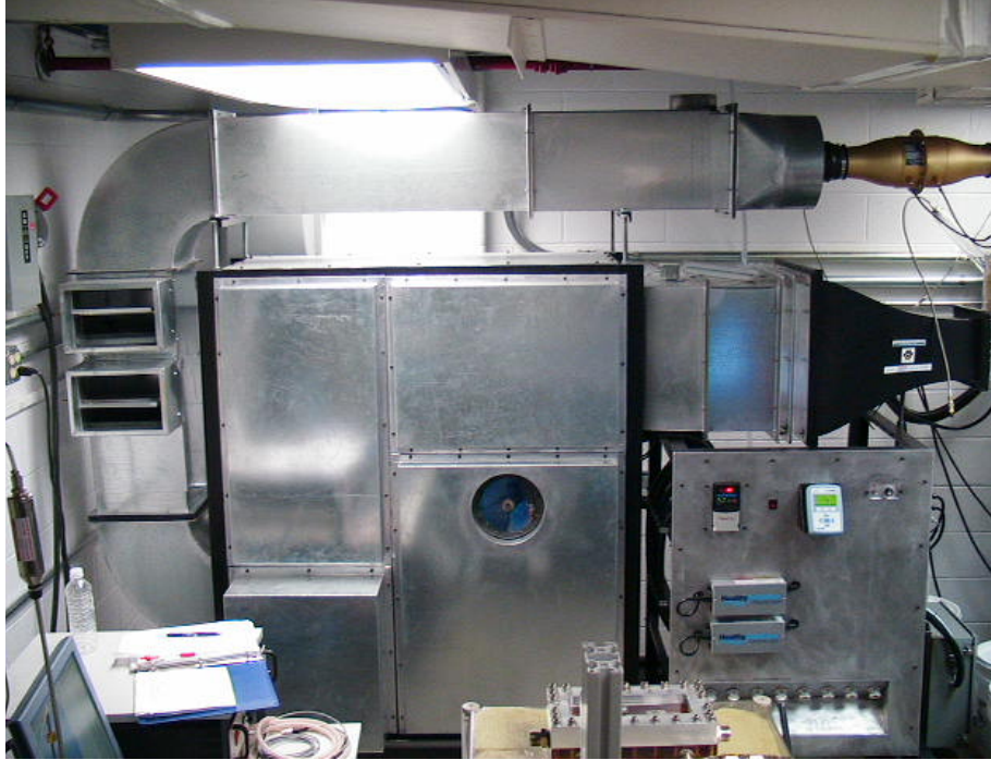
Figure 12 New and current air handler.
