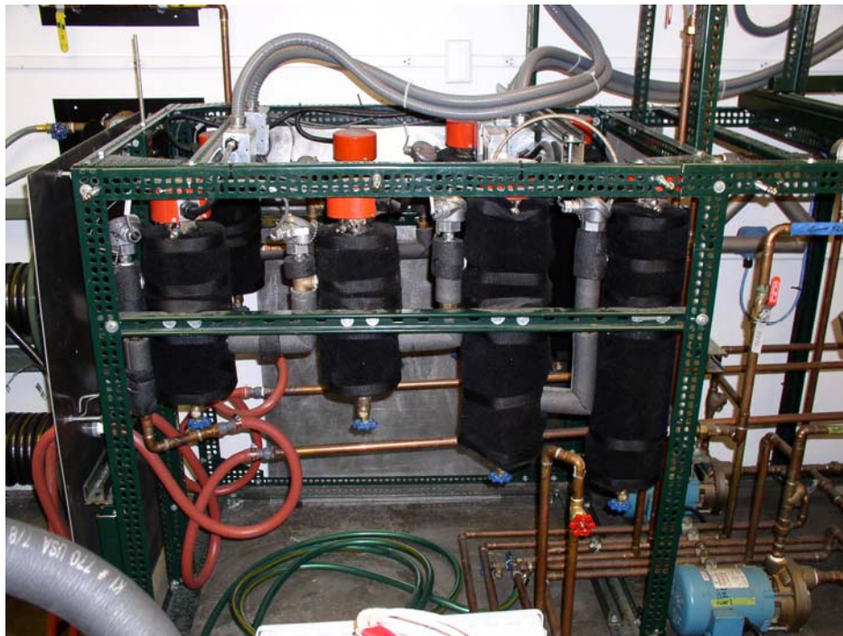
Figure 15 Watlow® resistive heaters (1 kW, 3kW, 6kW, and 7.5kW) in the Air Handler Conditioning Loop.
