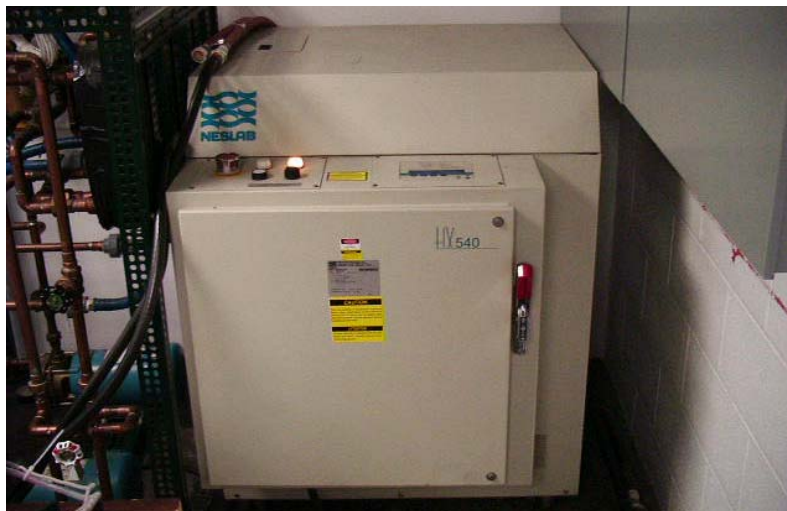
Figure 17 HX540 NESLAB® chiller used for supplement cooling for Air Handler Conditioning Loop.
