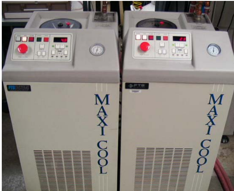
Figure 16 Maxi-Cool chillers used for supplement heating and cooling for Air Handler Conditioning Loop and Refrigerant Loop.
