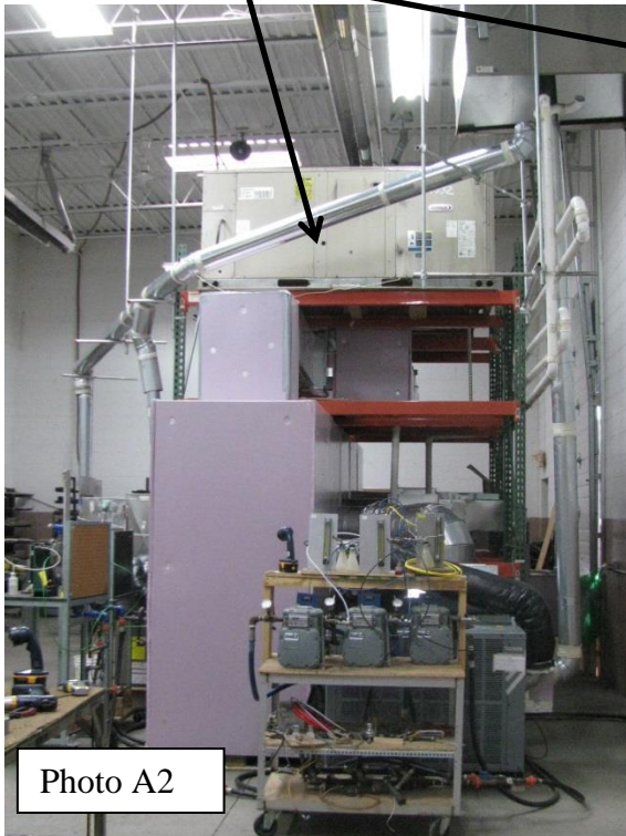
2 of 4 Air Conditioning Systems Mounted Above Air Duct Chambers
