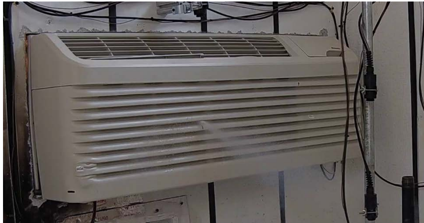
Figure 289 – PTAC_13 Discharge showing accumulation of liquid propane on the PTAC grill
