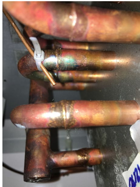
Figure 60 – Capillary tube as installed on the three door cooler evaporator
