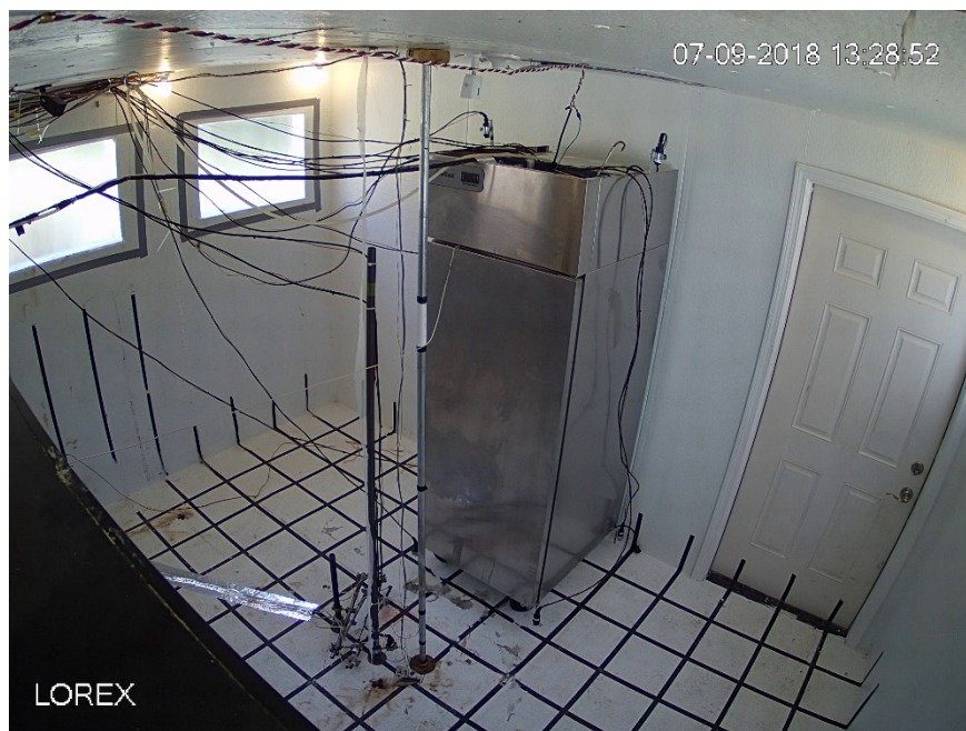
Figure 63 – Single door refrigerator installation
