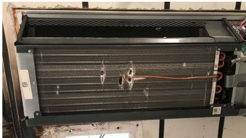
Figure 32 – ¼ inch discharge tube in the center of the PTAC evaporator coil
