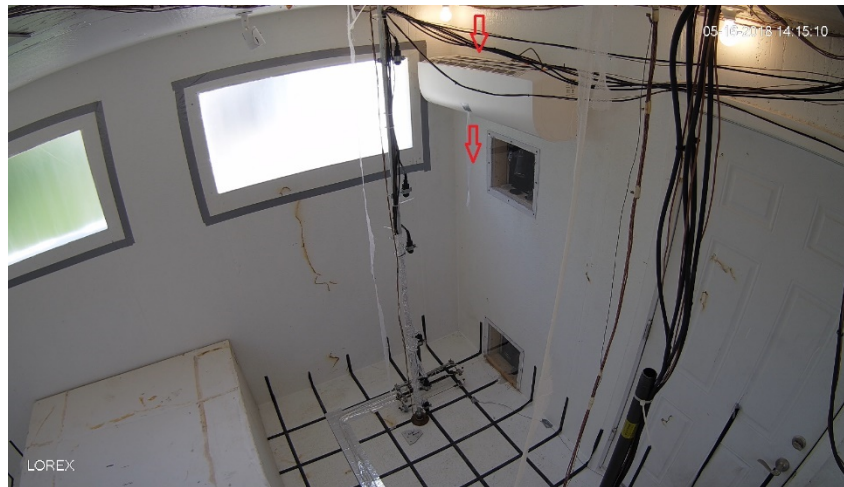
Figure 44 – Mini-split shown in location prior to a test. Red arrows showing the air flow path
