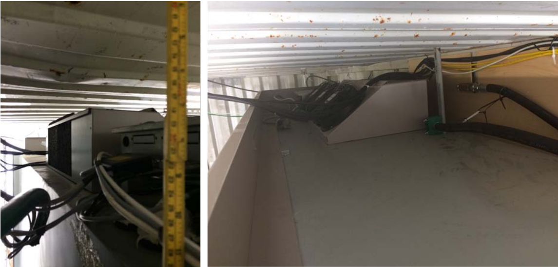
Figure 4.3: Condensing unit enclosure on the display case used in the test setup.
