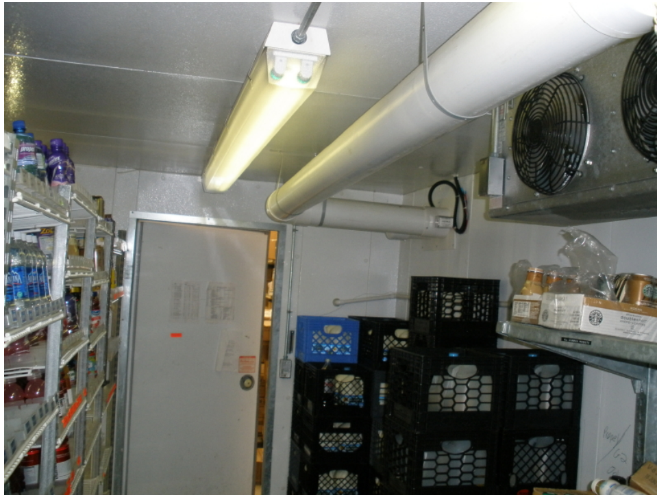
Figure 7. Photograph of the Interior of the 11-Door Display Walk-In Cooler at Tedeschi Food Shop (#110), Bridgewater, MA, looking from the Wall Opposite of the Personnel Door.
