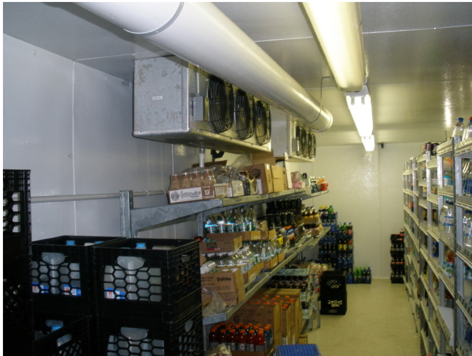
Figure 6. Photograph of the Interior of the 11-Door Display Walk-In Cooler at Tedeschi Food Shop (#110), Bridgewater, MA, looking from the Personnel Door.
