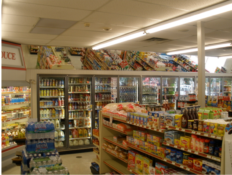
Figure 5. Photograph of the Exterior of the 11-Door Display Walk-In Cooler at Tedeschi Food Shop (#110), Bridgewater, MA.
