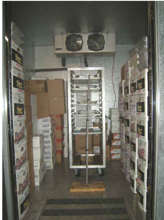
Figure 10. Photograph of Walk-In Freezer Tested by FSTC.
