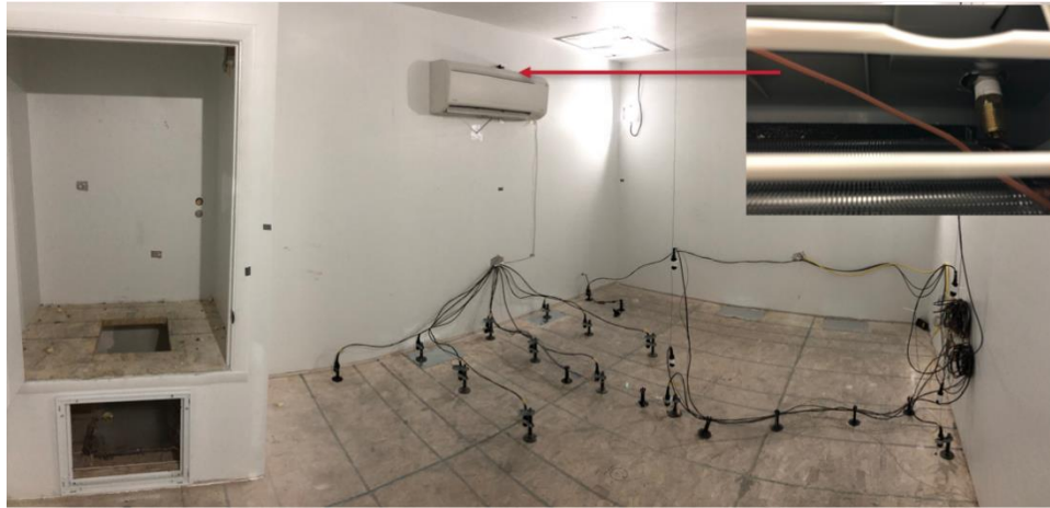
Figure 1 - Ductless Unit and Leak Location
