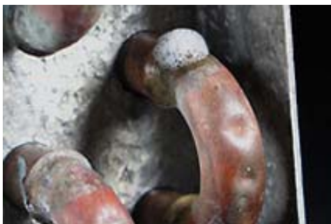
(a) Micro leak
