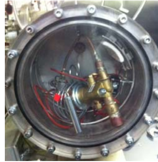
Figure 4.28: TXV n°1 installed inside the accumulation volume.
