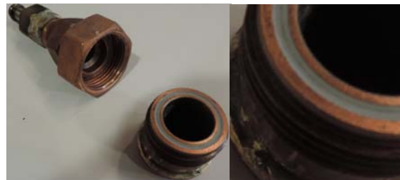
Figure 4.55: Rotolock fitting after cleaning.
