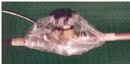
Figure 2.43: Example of a valve wrapped in a vinyl sheet [CLODIC 1998].
